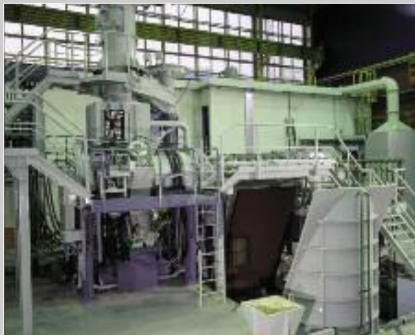
View with open casting chamber
