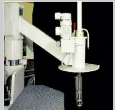
The revolver on the furnace lid enables charging, temperature measurement, sampling without interrupting the furnace atmosphere
